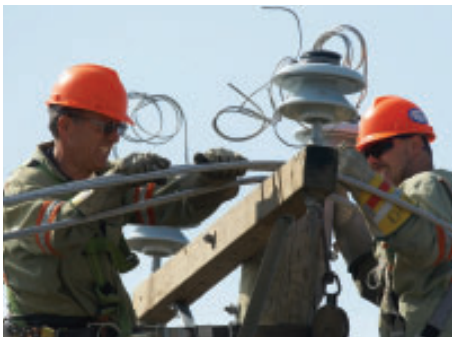
Figure 3 These workers are installing new wires and insulators on this hydro pole.
