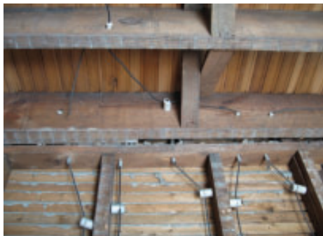
Figure 2 Knob and tube wiring was common in homes up to about 1930.
