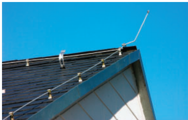
Figure 5 The lightning rod on this home directs any lightning strikes safely into the ground.
